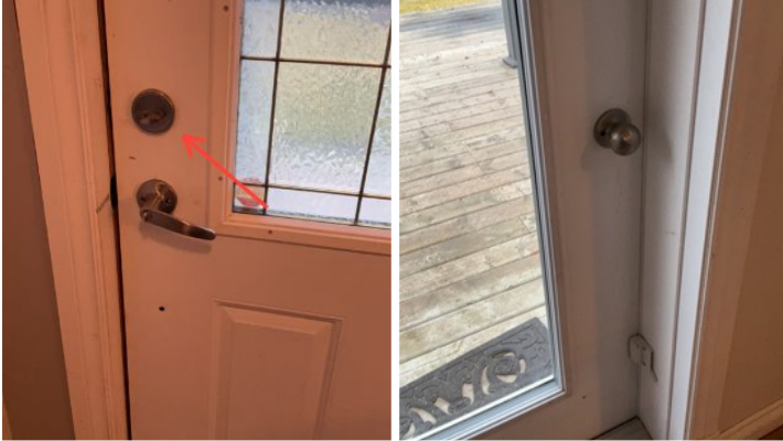
Recommend locking handle be installed
